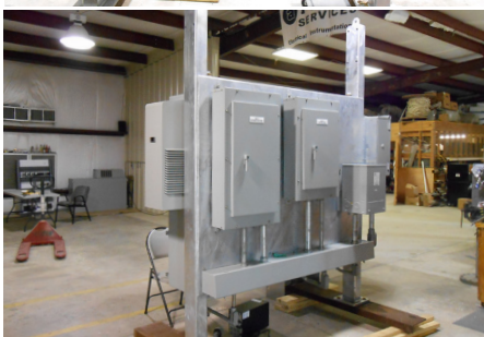
PLC PANEL ON SWITCH RACK – PIPELINE LOCATION
